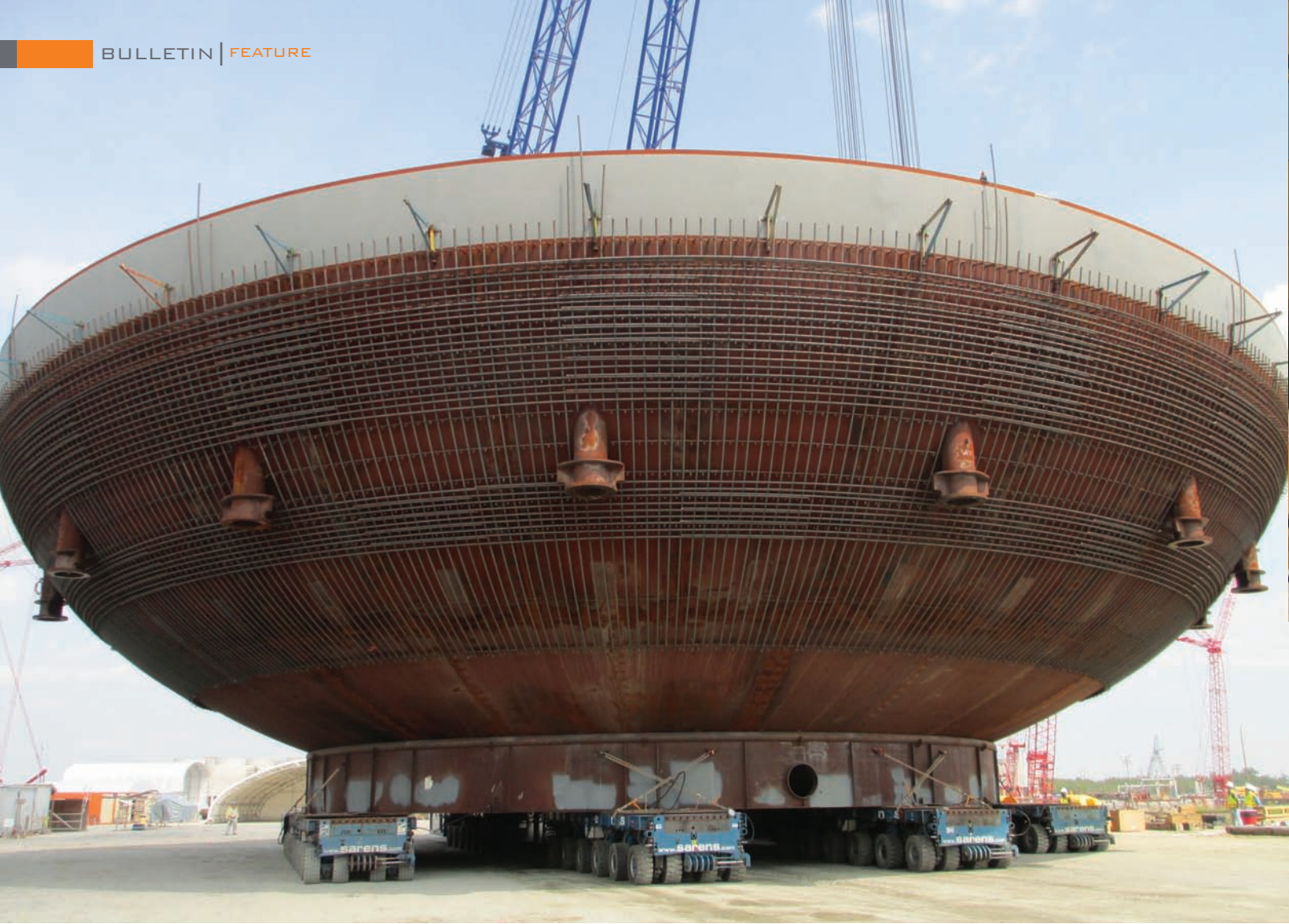
Close-up of the CVBH being placed on the basemat of V.C. Summer Unit 3. Photo courtesy of SCE&G.
