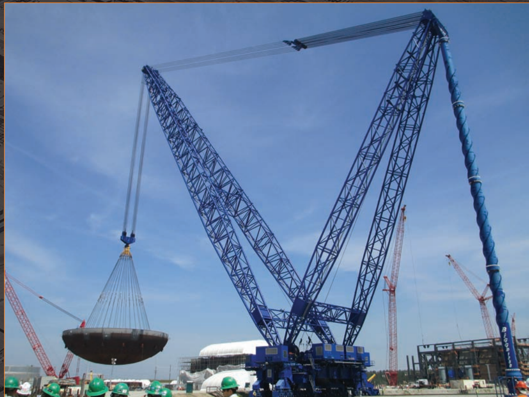
The containment vessel bottom head (CVBH) is placed on the basemat of V.C. Summer Unit 3 in May 2014. The approximately 900-ton CVBH was lifted into place with the Heavy Lift Derrick, which is one of the world's largest cranes. Photo courtesy of SCE&G.
